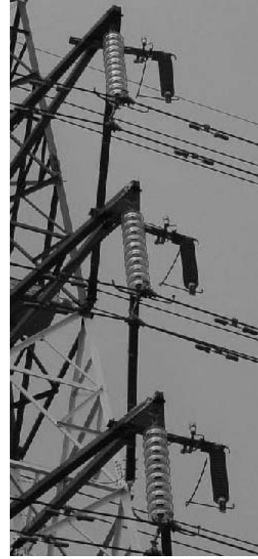
Fig.2 - Line surge arrester with an external gap installed on one 132 kV circuit
