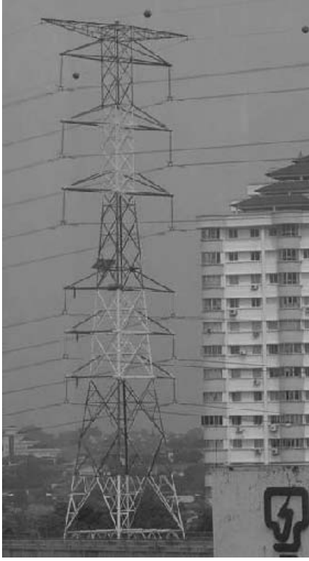
Fig.1 - Quadruple circuit transmission line 2 x 275 kV (top) and 2 x 132 kV (bottom)
